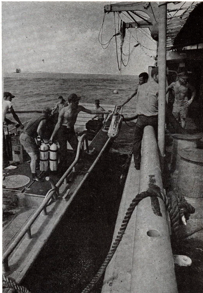
CURRENT divers load their gear on a utility boat in preparation for underwater repair job (below).
